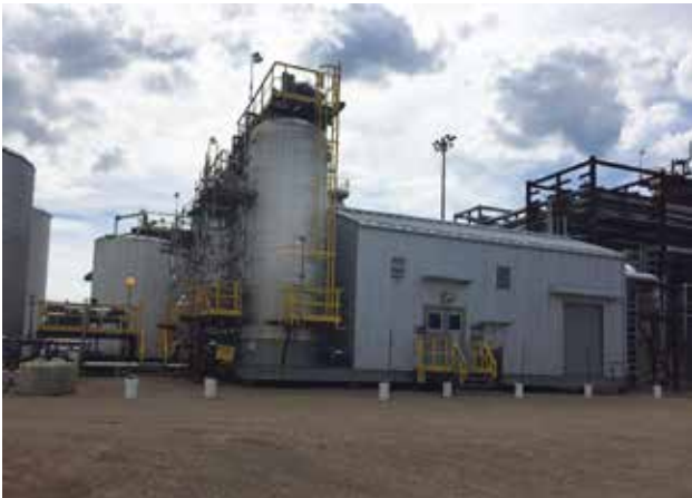
SAGD Sulfur Recovery Unit
