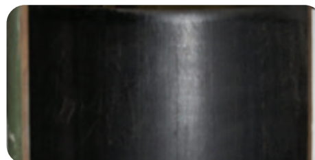
Segment of pipeline treated with PureCorr
