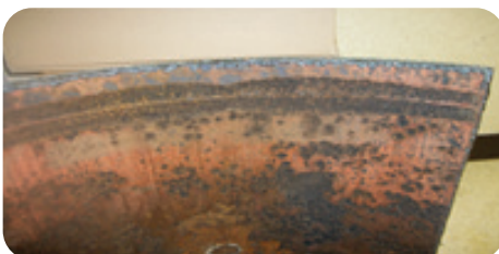
24" pipeline corrosion failure prior to application of PureCorr
